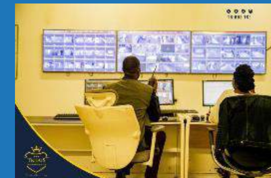
Security Operations Center
